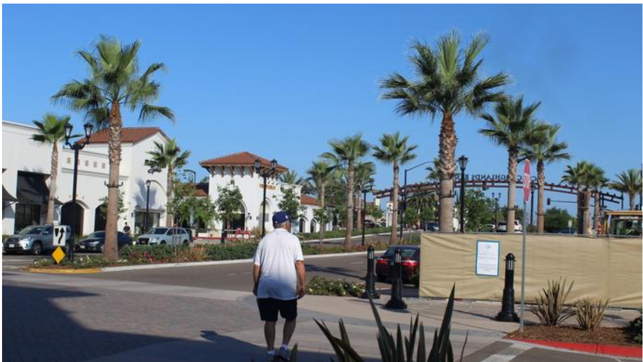
Construction has begun on new retail and service space as well as a new parking structure. (Karen Billing)
